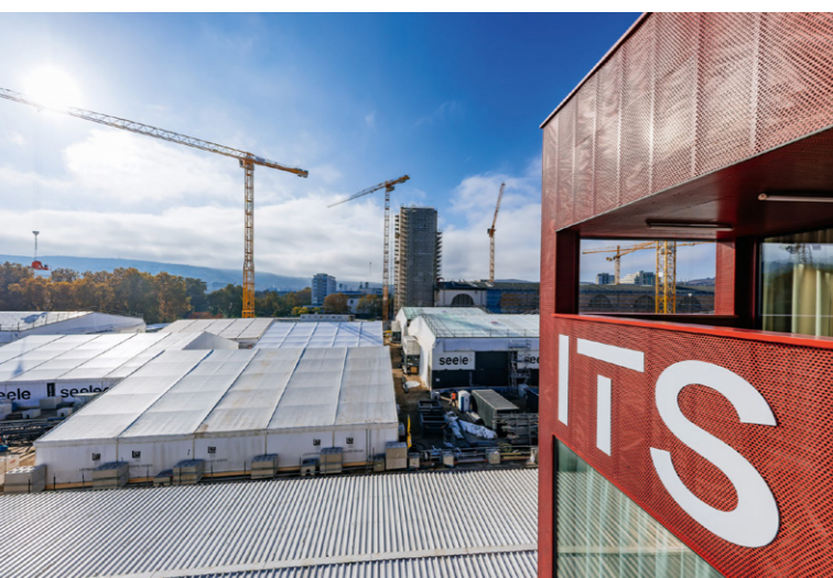
You couldn't get any closer to the action: the InfoTurmStuttgart is located right in the heart of the construction site.
